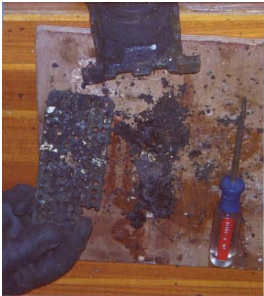
IT'S IMPORTANT TO REGULARLY CHECK YOUR BILGE PUMP STRAINERS AND CLEAR THE DEBRIS WHICH ACCUMULATES AS SHOWN IN THIS PICTURE OF ENVOY'S STRAINER.
