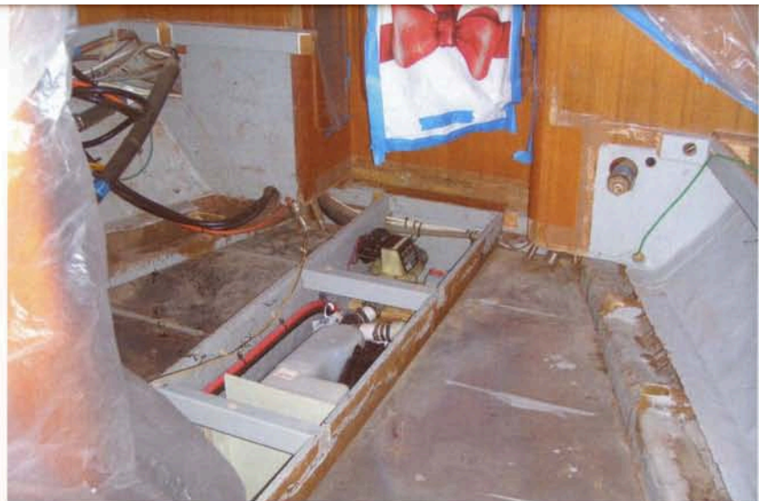
ENVOY'S GUEST CABIN AFTER STRIPPING OUT BUILT-IN FURNITURE, SHOWING THE WATER TANKS BEFORE THEY WERE REMOVED.
